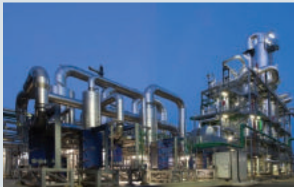
The new Mater-Biotech bio-BDO plant is now onstream at Bottrighe, with a capacity of 30,000 tonnes/year
